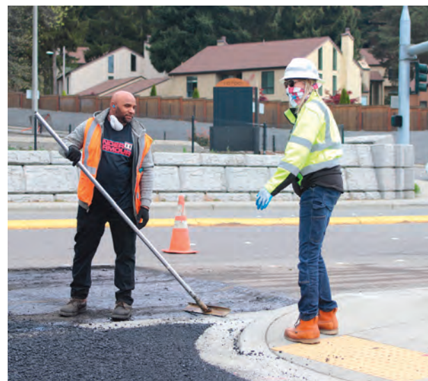
Cheryl Dowse, a right-of-way inspector, improvises personal protective gear as she monitors street construction.
